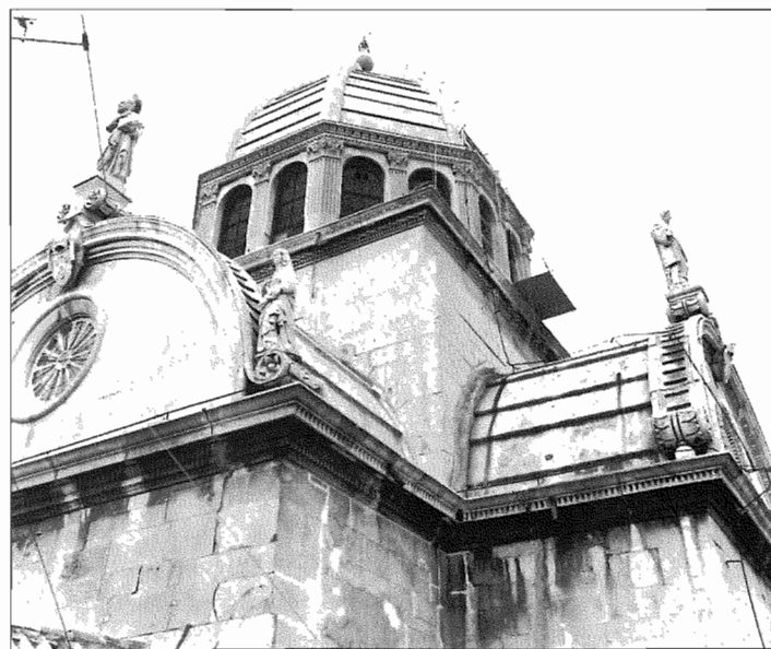
17 Tragovi curenja kišnice kroz loše zabrtvljene reške između elemenata kamenih žljebova (katedrala sv. Jakova u Šibeniku) Cases of the trickling of rainwater through poorly sealed joints between the elements of stone guttering (St James' Cathedral, Šibenik).
